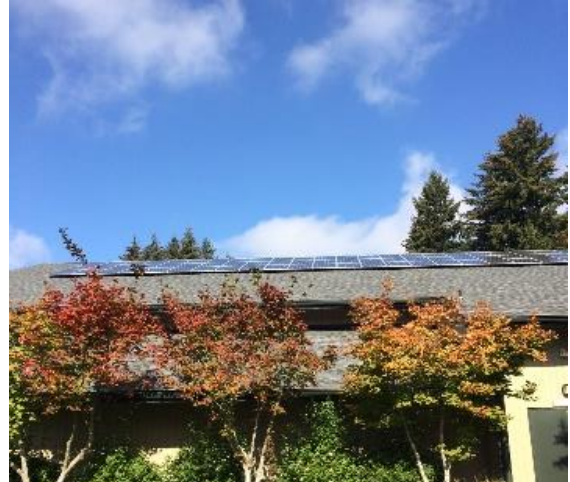
Photo: Crossroads Community Center Solar Array
